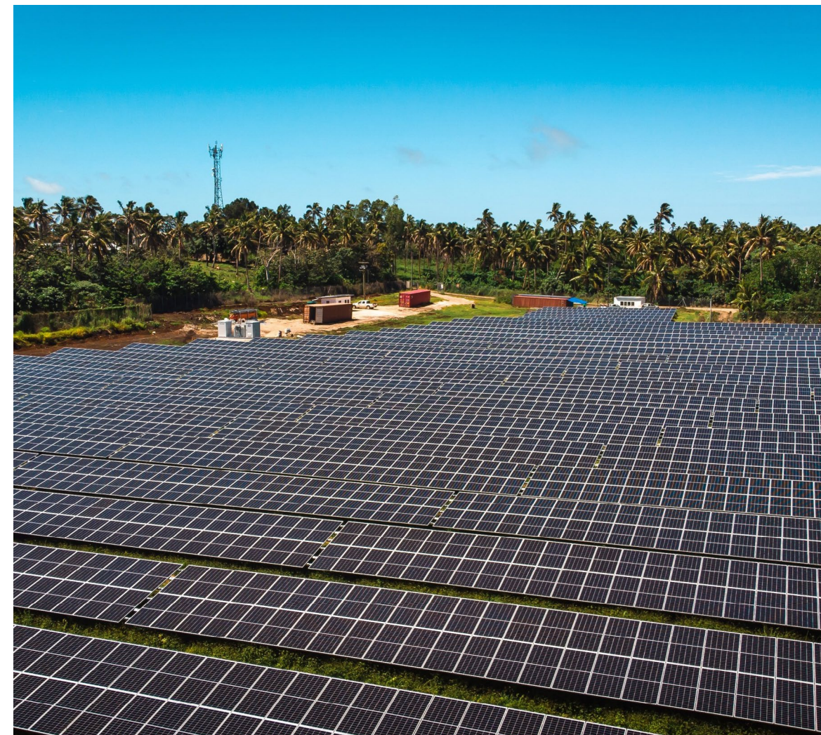
Right: One of Sunergise International's solar installations in Tonga
