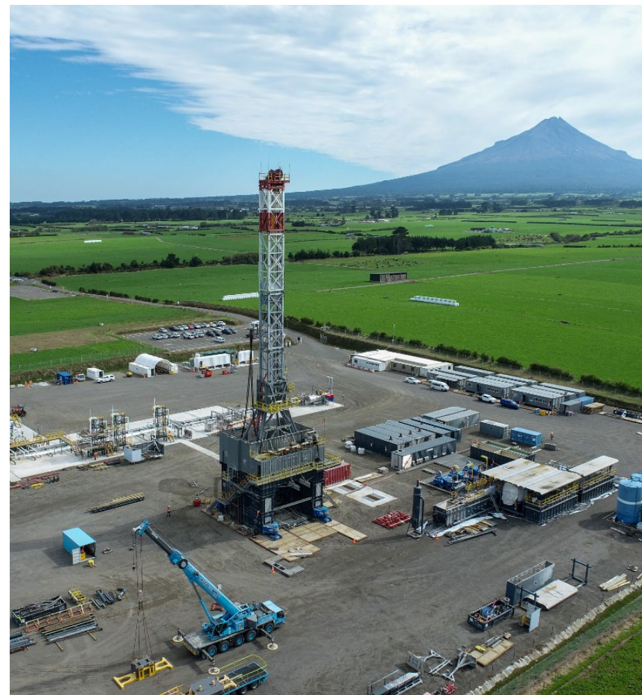
Above: The Big Ben rig at the Kapuni J wellsite in South Taranaki
