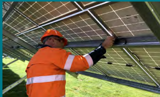
A Nova Energy employee checking the solar panels at the Kapuni Solar Plant in South Taranaki.
