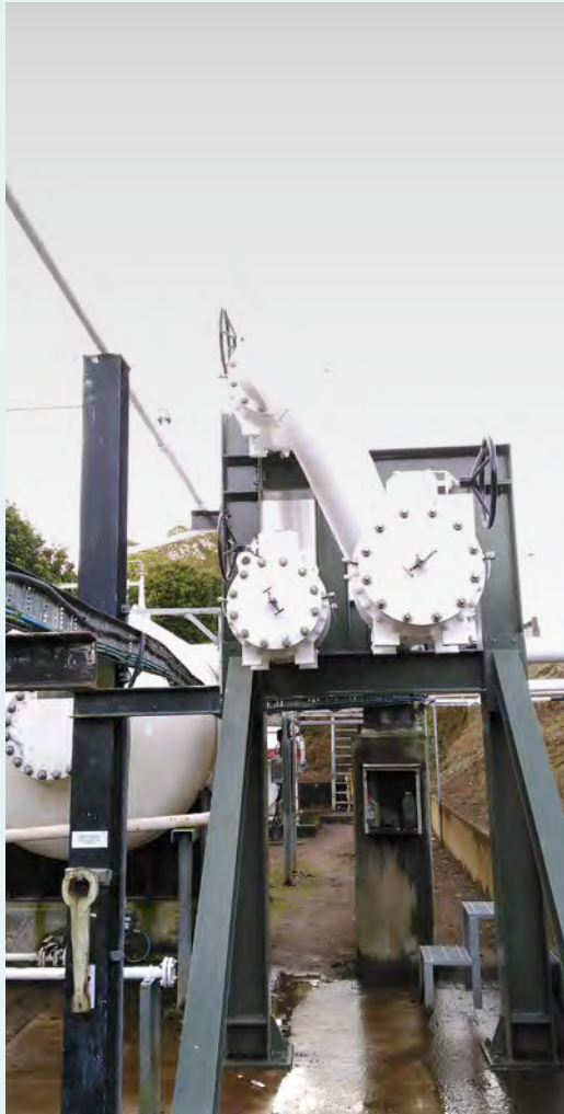
The tie-in valves installed on pipelines at KGTP in 2022.
